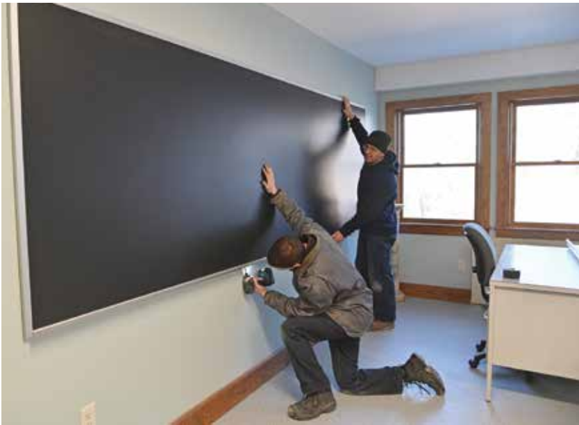
Above: Brother Gerard and Brother Anthony Marie install a new chalkboard in what will be the new 5th grade classroom.
